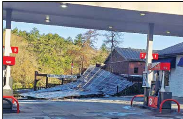
One of the roofs on Main Street Nursery blew off and landed at the gas station next door and knocked down power lines. - Photo by Kim Lewicki
